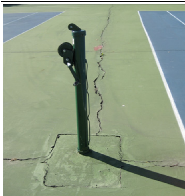
Cracked pavement at the Windemere Park tennis court. (Image provided by city staff in a slide presentation to PAC.)
