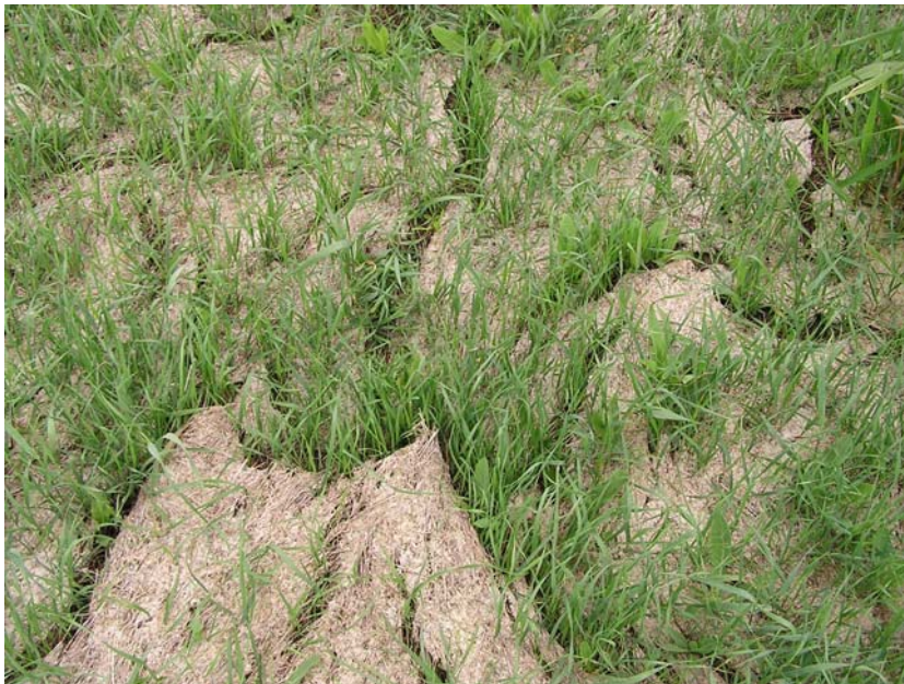
Photo 2. Evidence of rodent tunneling near east end of Runway 24. 6-10-09.
