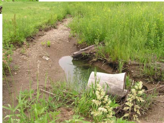
Photos 4 and 5. Drainage ditch on south end of project where it emerges from culvert. 6-10-09.
